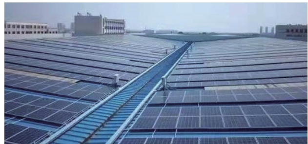
Roof Photovoltaic Power Generation
