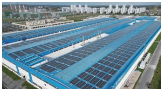
Photovoltaic power generation
